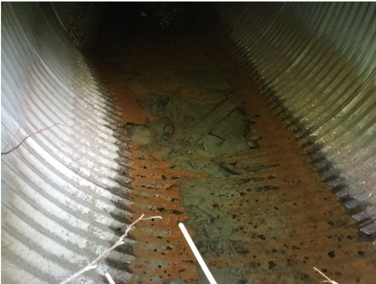
Upchain culvert corroded without a floor at inlet
